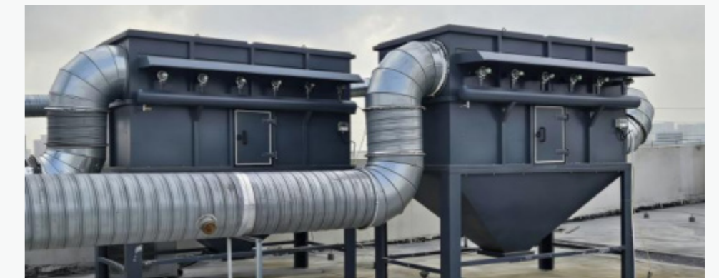
Newly Added Waste Gas Filters at Wuxi Manufacturing Base, Jiangsu
